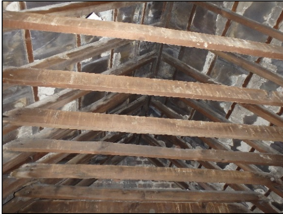
Figure 5.7.13: Attic space of Georgian building with unlined slates, which contained a large proportion of bird droppings and a Feral Pigeon.
