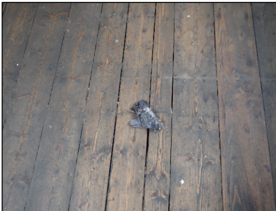
Figure 5.7.14: Dead Feral Pigeon, located on the second floor of a Georgian building.
