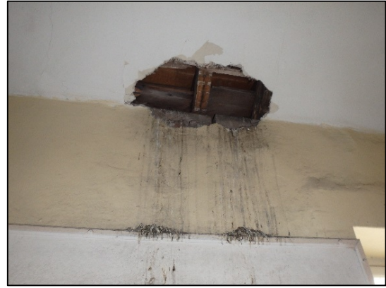
Figure 5.7.15: Example of a hole in the ceiling exposing limited section of attic space and bird droppings beneath.
