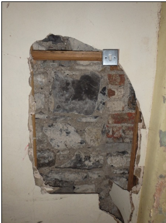
Figure 5.7.10: Gaps between insulation boards and wall, located in basement of Georgian building.
