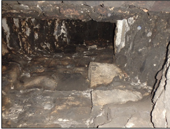
Figure 5.7.9: Interior of chimney suitable for roosting bats, located in basement of Georgian building.
